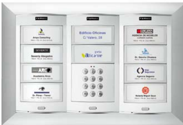
office directory with access control system by keypad
